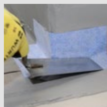
Bed MC-FastTape AE (buitenhoek) of MC-FastTape IE (binnenhoek) in de verse eerste laag in.
